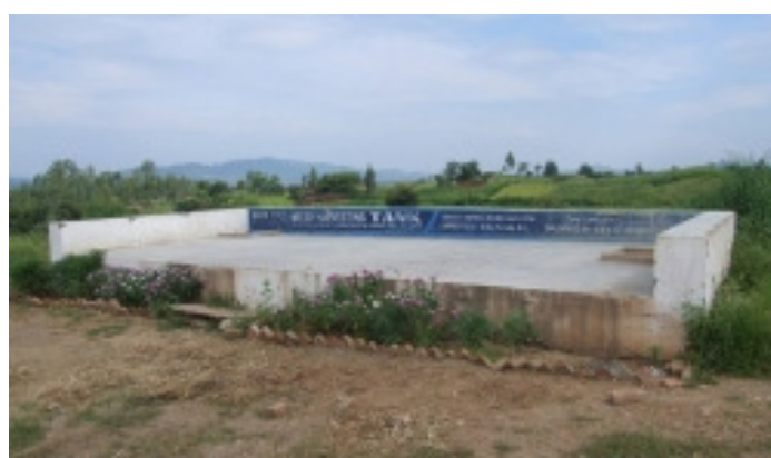
The roof rainwater harvesting tank at Beeda school
